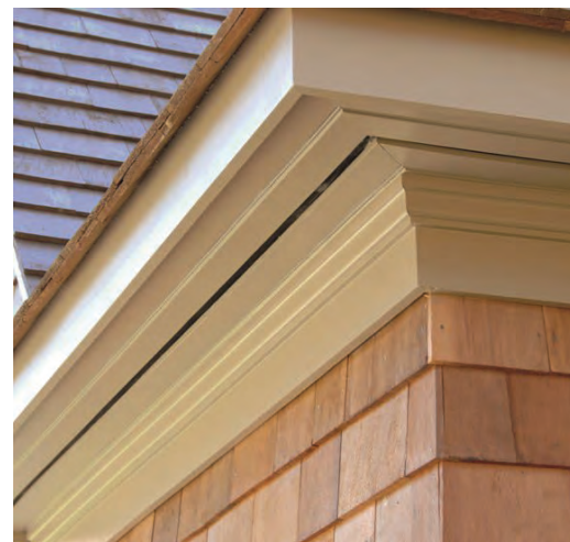
Figure 3.14 (PP): A continuous vent is tastefully incorporated into the design of the soffit for a hipped roof. The vent provides ventilation to the attic and has been designed to accent the molding and trim work.
