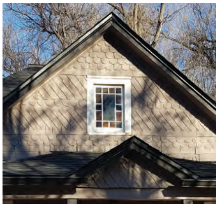
Figure 4.12 (PP): Shakes in various shapes employed in a historic building, Longmont, Colorado.
