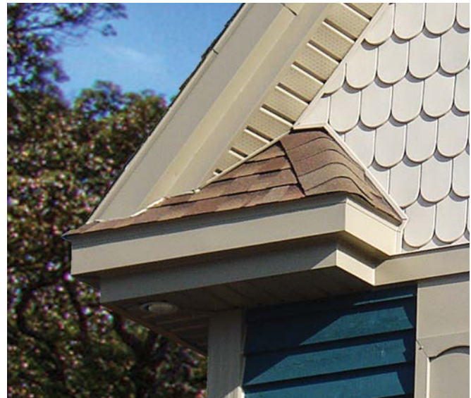
Figure 118: The eave return, shown here with vinyl siding, soffit, and aluminum fascia, terminates the roofline with a more accurate, traditional detail.
