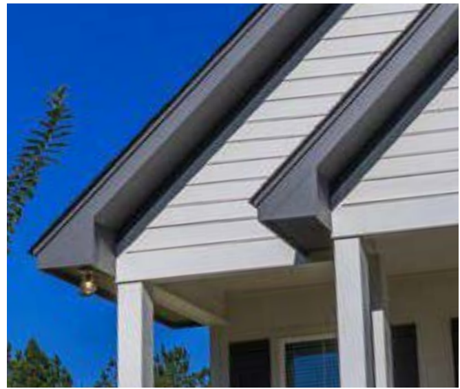
Figure 116: Affectionately known as the "pork chop," this style of eave termination came courtesy of truss roof construction as a way to finish the end of the rake at the soffit corner.
