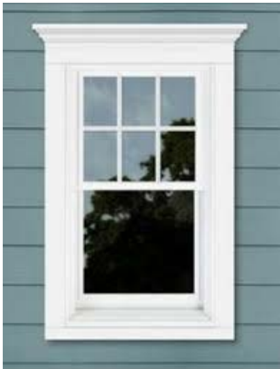
Figure 76: Vinyl window casing with an integrated pocket, or rabbet, to receive siding looks appealing when viewed from the street.
